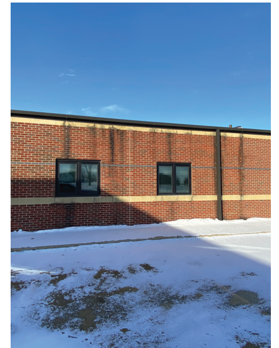
Staining at exterior masonry.
