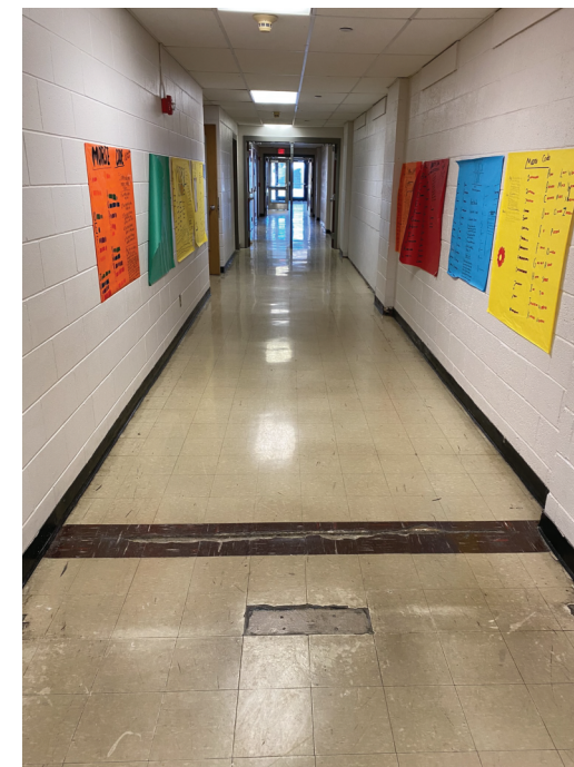
Poor condition corridor
