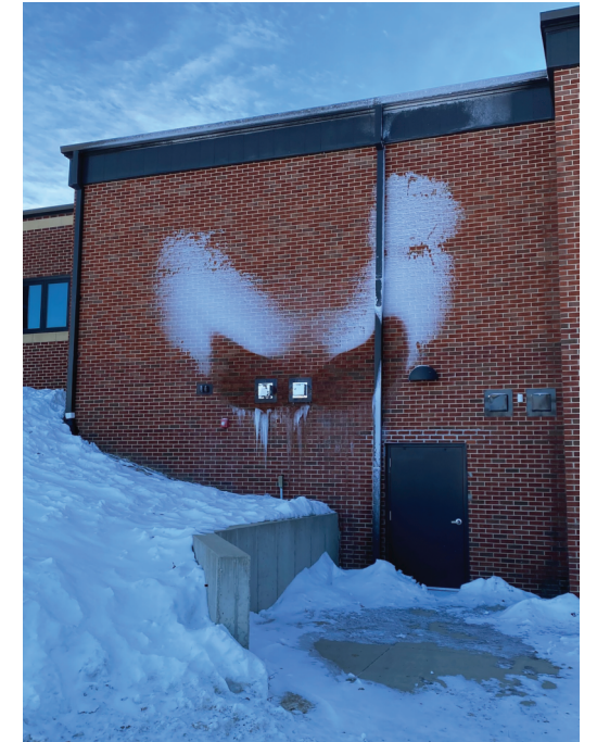
Exhaust condensation at exterior masonry.
